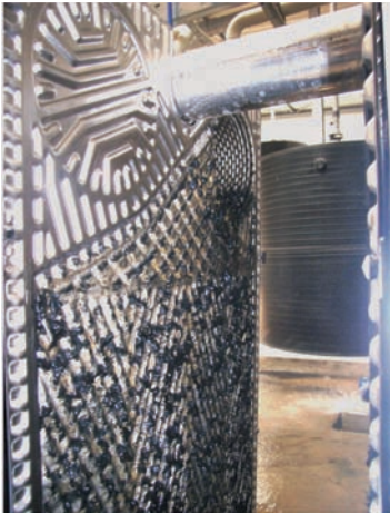
Fig. 18: Unprotected plate heat exchanger
