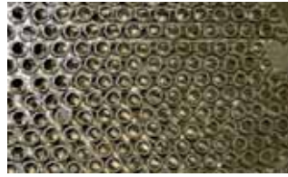
Same heat exchanger with 300 µm KAF-Filter. Inspection opening after 9 months
