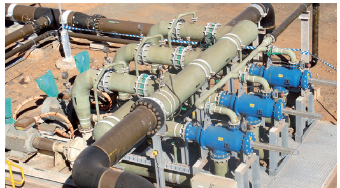
3 x 16"/DN 400 KAF® Filter – desalination
